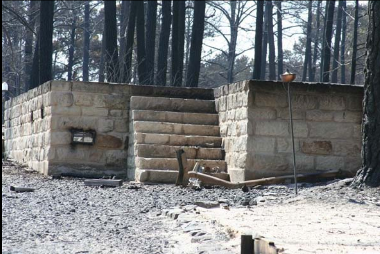
LOCAL, TDEM & FEMA DAMAGE ASSESSMENTS
